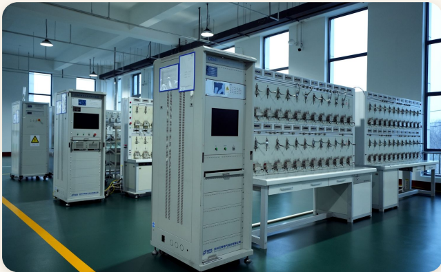
Single-phase meter verification
